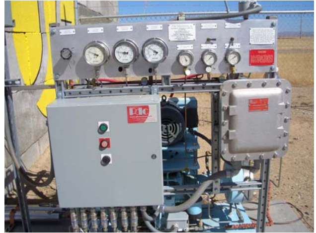
Figure 6. 3,000 psi Hydrogen Compressor Permission: Pdc Compressors; Source: ReliOn
