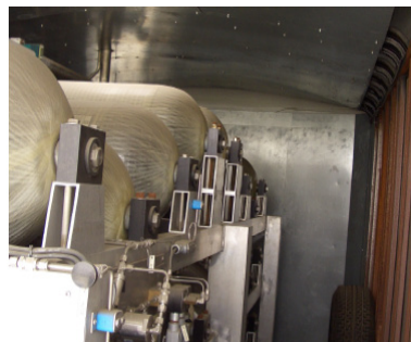
Figure 3. 2 kg (800 SCF) Composite Pressure Vessels Mounted In Hydrogen Mobile Fueler Service Source: SCI Composites
